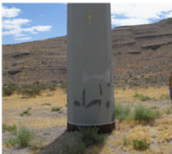
Pole 2: This is a close-up view of the second structure tested. It is a direct embedded pole set in concrete
