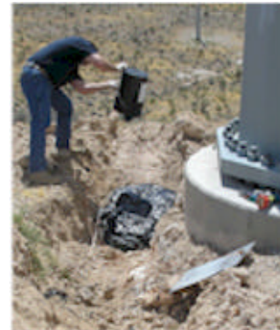
Pole 4: This photo shows a second kit being poured on top of the galvanized plate to insure maximum contact with the plate and to insure a water resistant seal to protect the plate from further degradation.
