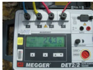
Pole 2: Normal, concrete backfilled pole with 10' x 3/4" copper ground rod. Reading is 24.3 ohms.
