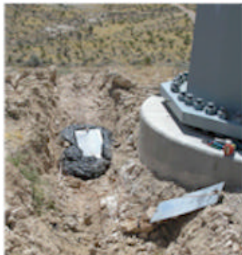
Pole 4: This is a photo showing the trench dug with a Poly-Ground® kit poured in the trench and the galvanized plate placed on top of the risina foam.
