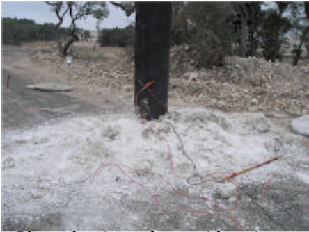
Photo showing pole set with native spoils with megger wires attached to ground rod.
