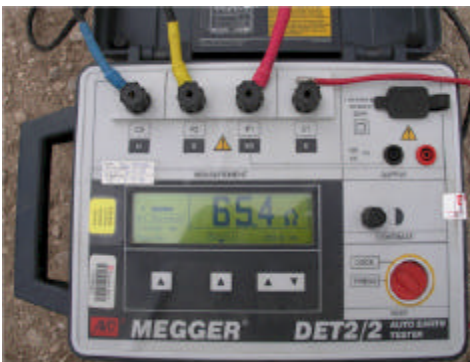
Photo showing final reading of the Poly-Ground installed pole. Reading is 65.4 ohms.
