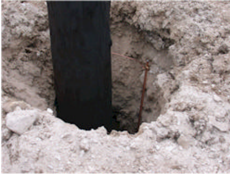
Close up of hole. Notice the location of the ground rod in the annular space
