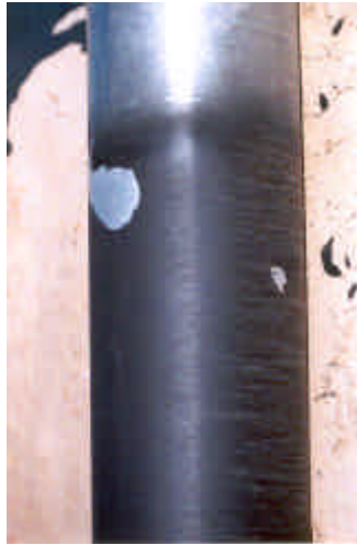
Pole showing Corro-Coat issues
